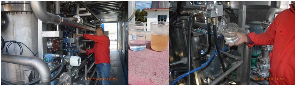
Left- Operator taking sample of raw water- Two Membrane Housings 12.5 m 3 /hr each Right- Operator taking sample of permeate from Membrane housing 1
