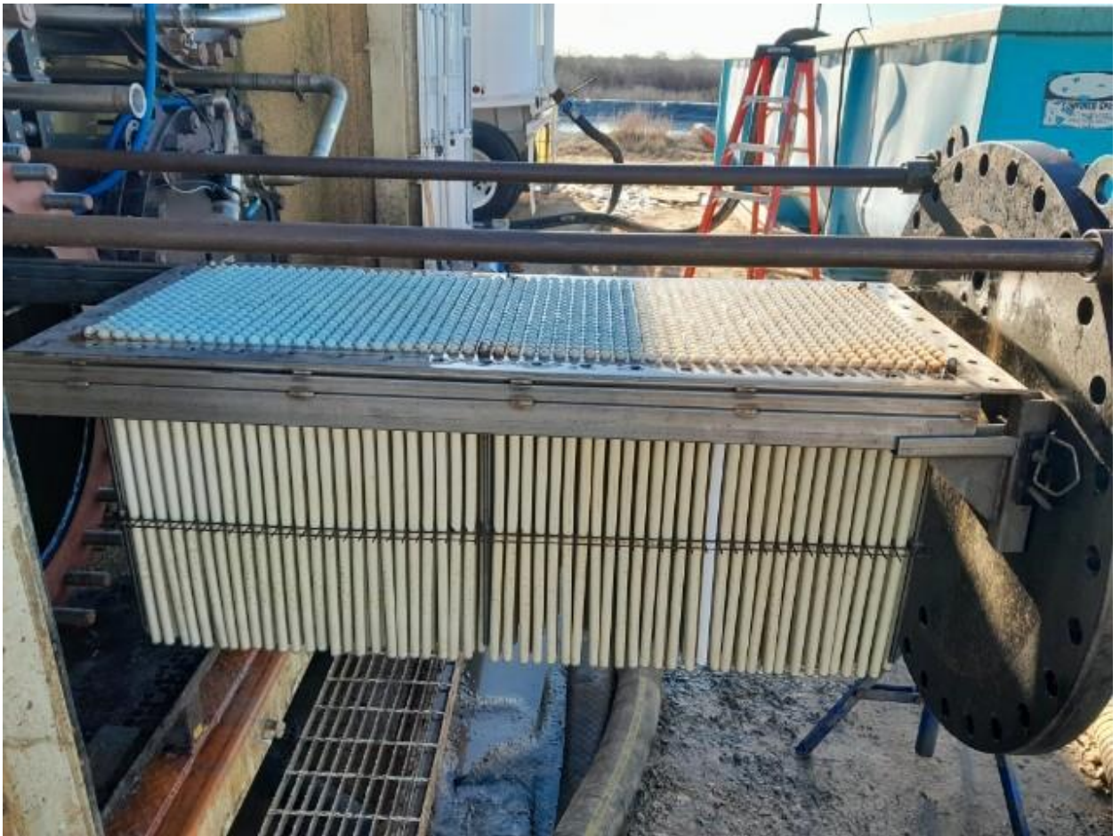
Figure 25 The Replaceable skin layer membranes after two months of operation with the slide out tray for easy maintenance.
