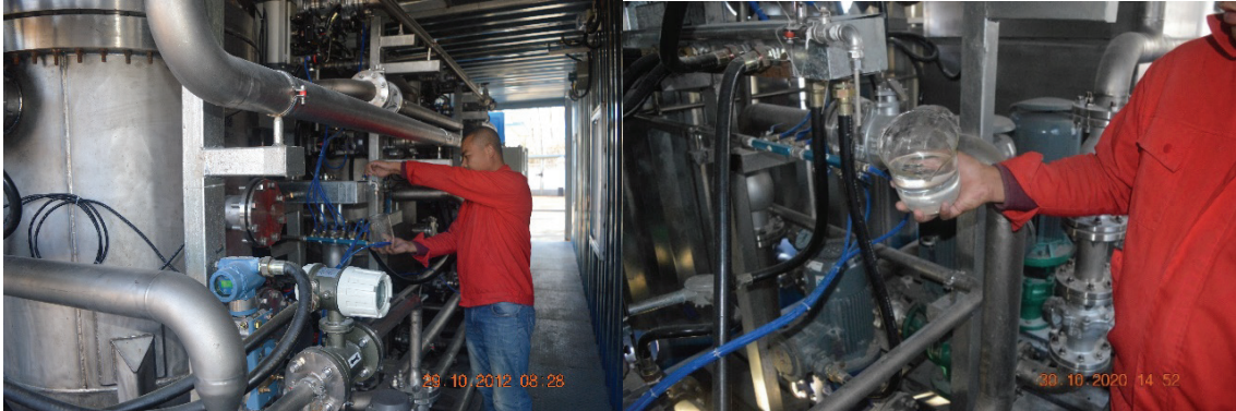
Figure 8: Dajing China: Operators taking samples on 25 m 3 /hr Replaceable Skin Layer Membrane.
