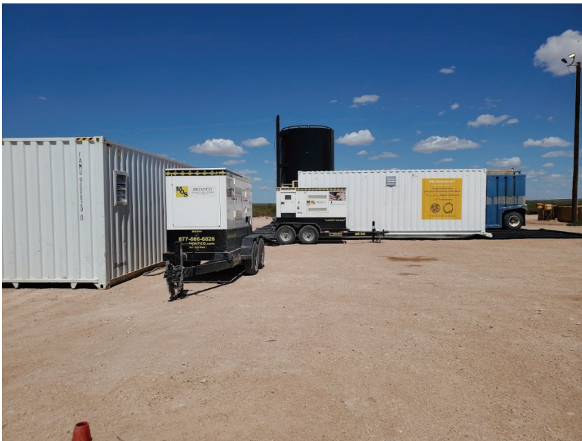
Figure 21 Setting up Replaceable skin layer membranes Sea Container unit at SWD Facility – Barstow TX
